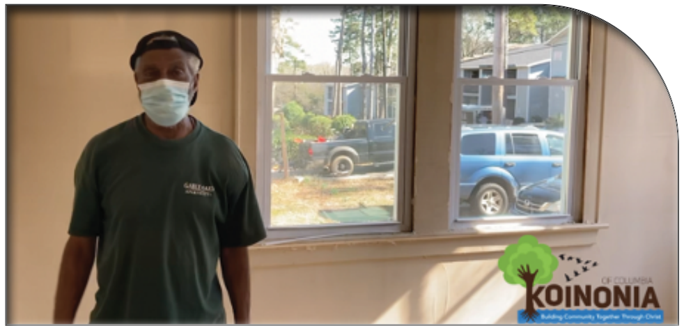
Larry Harden shows the carpentry and plumbing renovations he's completed at Koinonia's house as part of the missions report at the 2021 virtual General Assembly.
